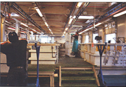
Figure 4. A view of the anodizing tanks inside P.K. Selective's warehouse.
